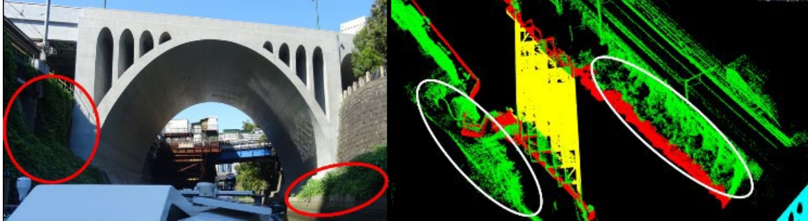
Figure 9: Area where vegetation covers the revetments (near Hijiribashi Bridge).
